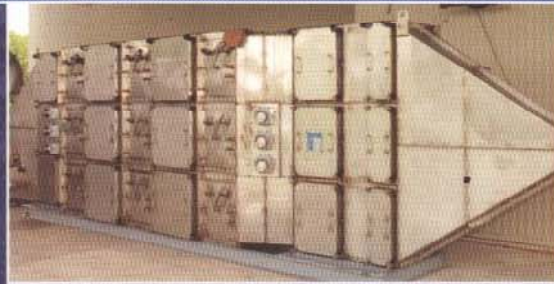
Sophisticated air monitoring and filtration system protects workers and the environment.
